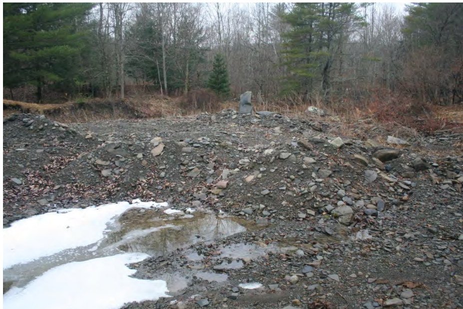
Main Branch at STA 46+00 Eroding bank March 7, 2017
