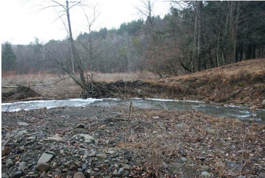
Main Branch at STA 46+50 Eroding bank March 7, 2017
