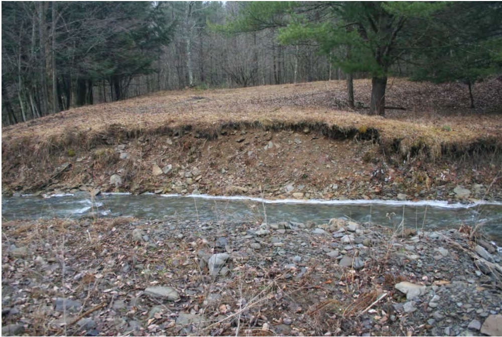
Main Branch at STA 46+50 Eroding bank March 7, 2017
