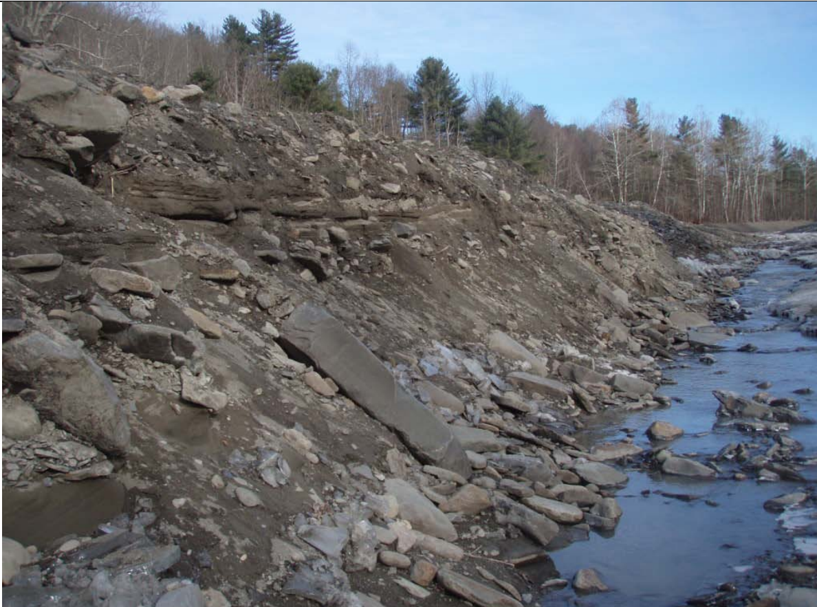
Photo 51: Close-up of loose bank material on right bank
