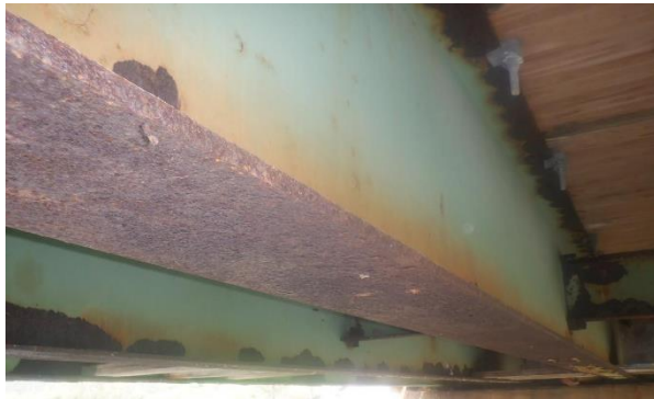
Figure A: Failed paint on the structural beam
